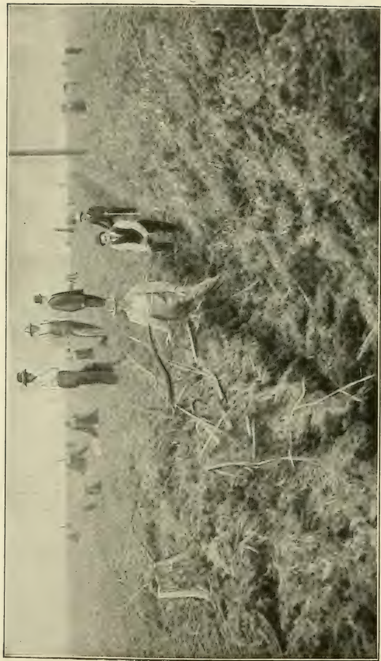
A DITCH BLASTED WITH DYNAMITE—WILL SQUARE UP AS SOON AS FILLED WITH WATER
